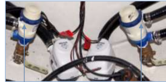
Pumps To Fill Valves
