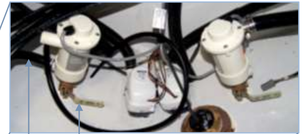
Shut Off Valve
