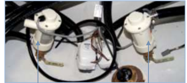
Pumps To Fill Valves
