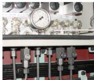
Fig.3) Damper and pressure gauge
