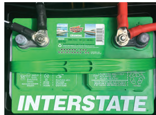
Battery post connections
