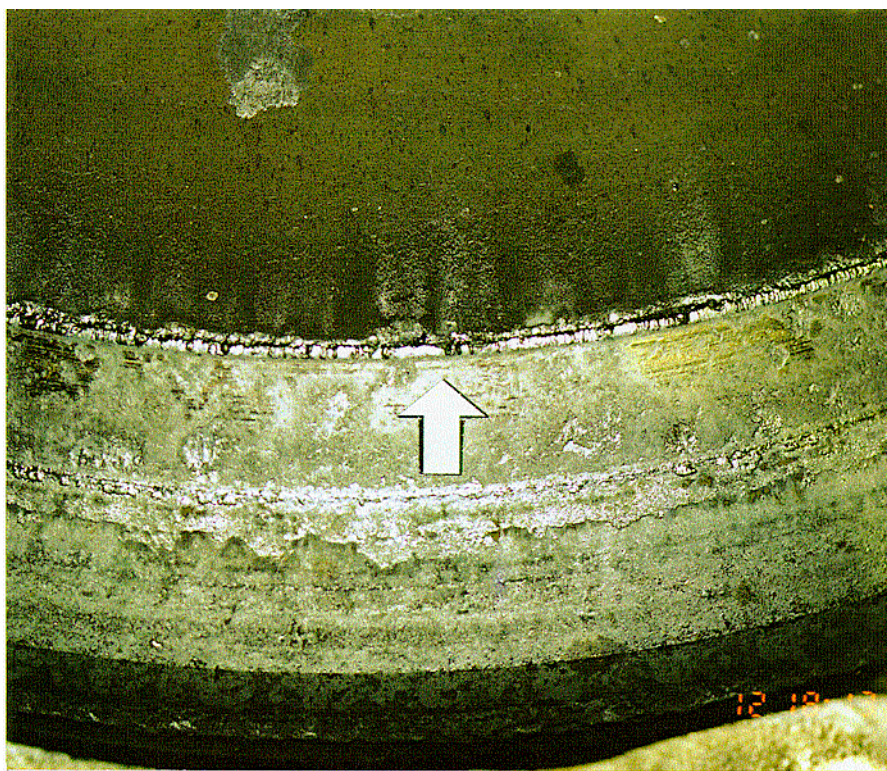
Photo 2: Minor leakages, and “fans”
