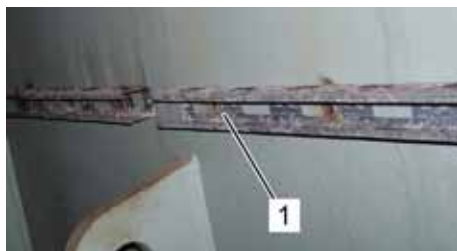
Fig. 68: Cable trays on engine block
