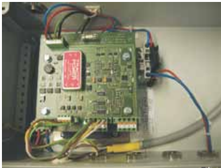
Fig. 12: Line Converter box type GHG02611-4 opened
