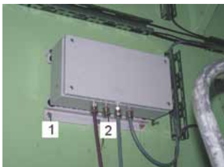
Fig. 63: Mounting Line Converter box
