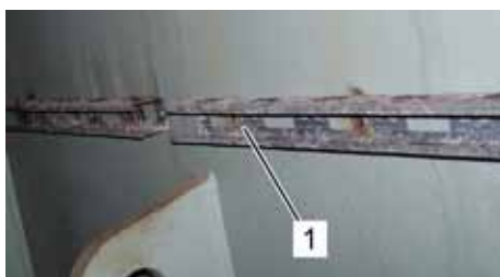
Fig. 82: Cable trays on engine block
