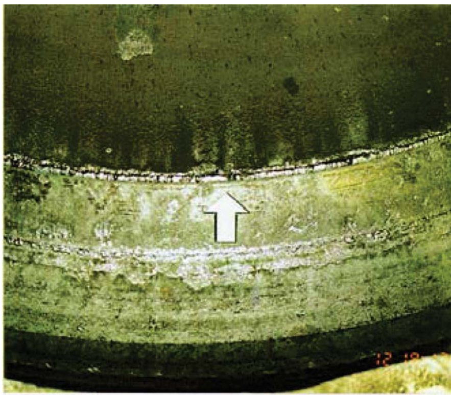
Photo 2: Minor leakages, and “fans”
