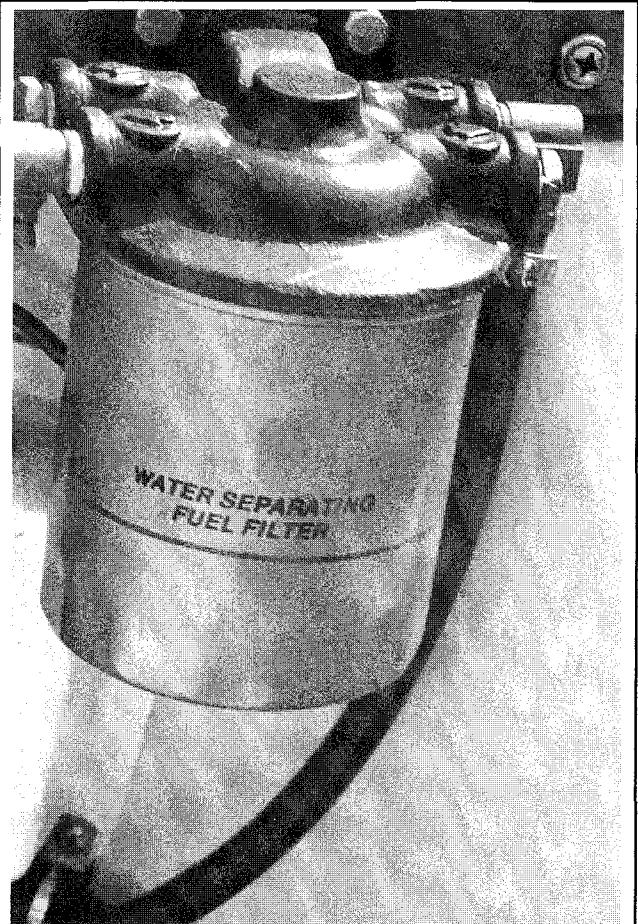
Fig. 89 A water separating fuel filter installed inside the boat on the transom
