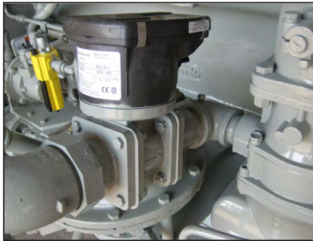
Figure 16-2: Fuel Control Valve
