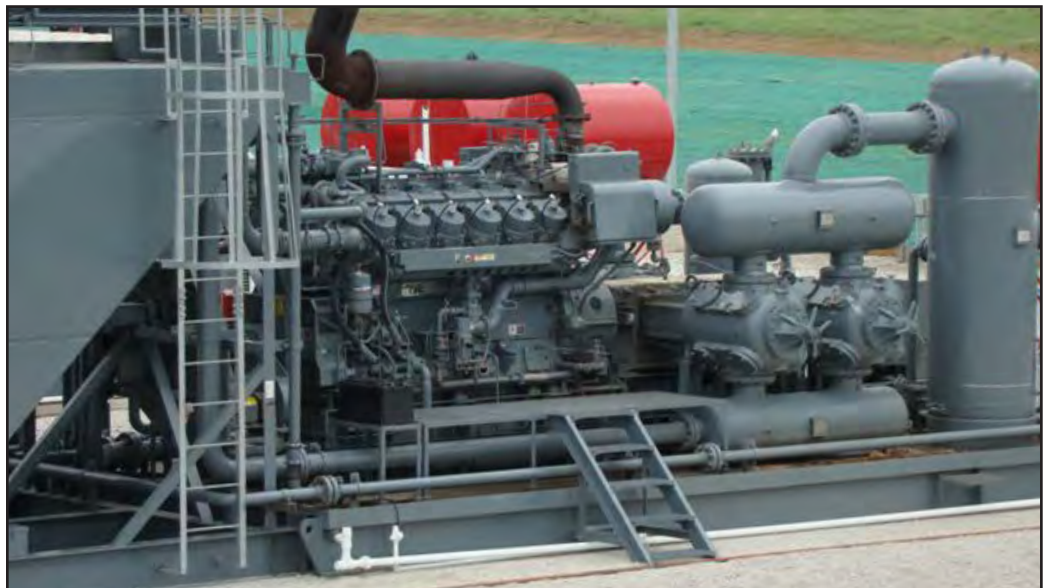
Figure 23-2: Engine Work Platform and Ladder for Access to Catalyst Element in Exhaust
