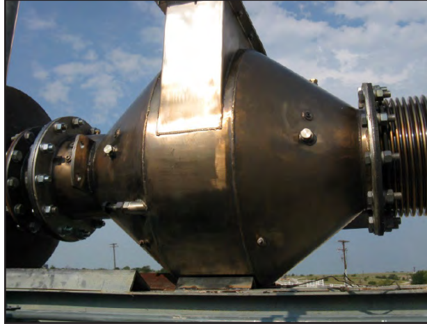
Figure 15-4: emPact catalyst installed
