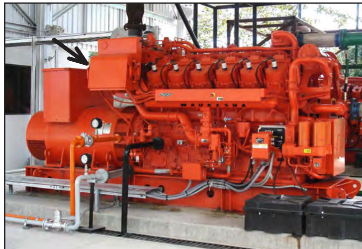
Figure 13-1: Standard air cleaner assembly mounted on a 12-Cylinder VHP
