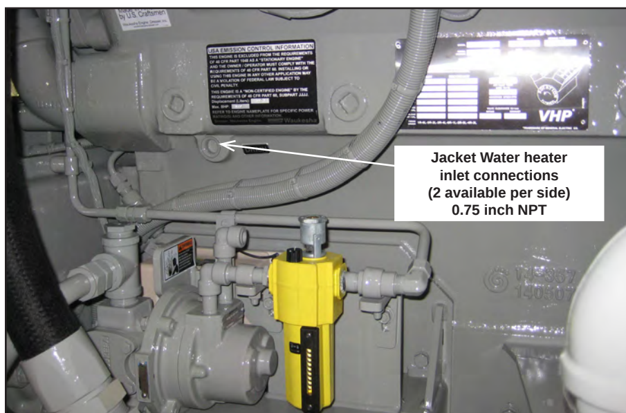
Figure 9-5: 12-Cylinder water heater outlet connection
