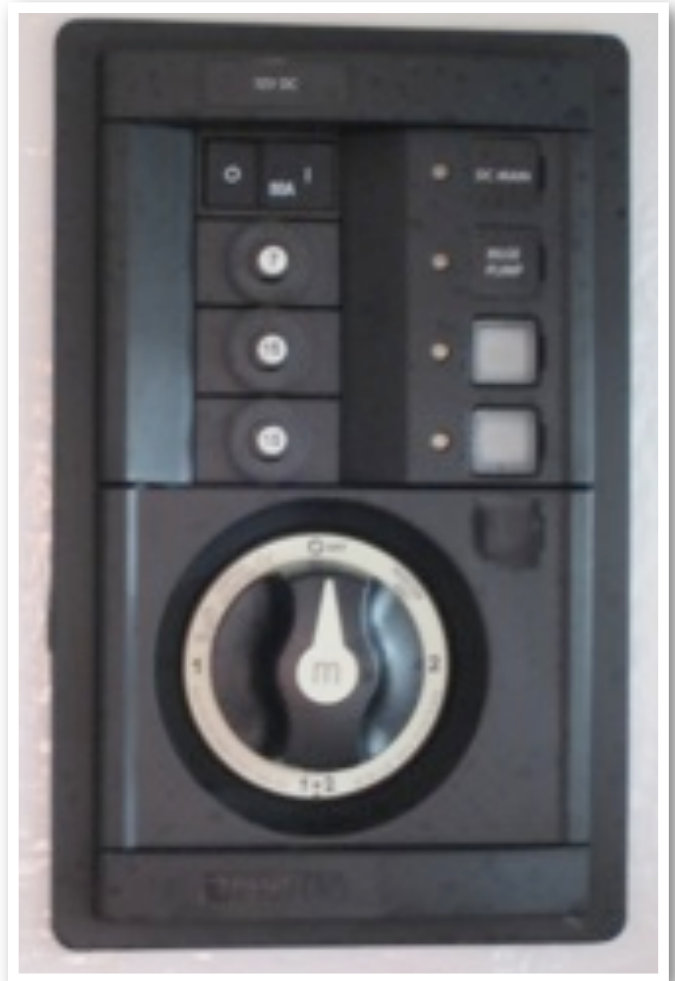
Battery Switch, Shown in the "Off" Position
