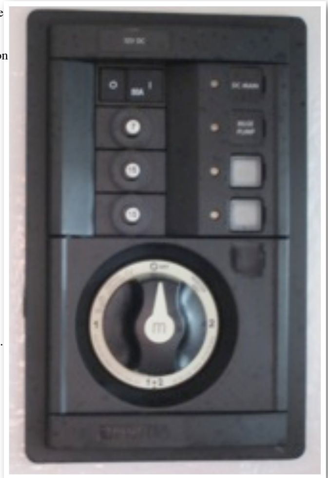
Battery Switch, Shown in the "Off" Position
