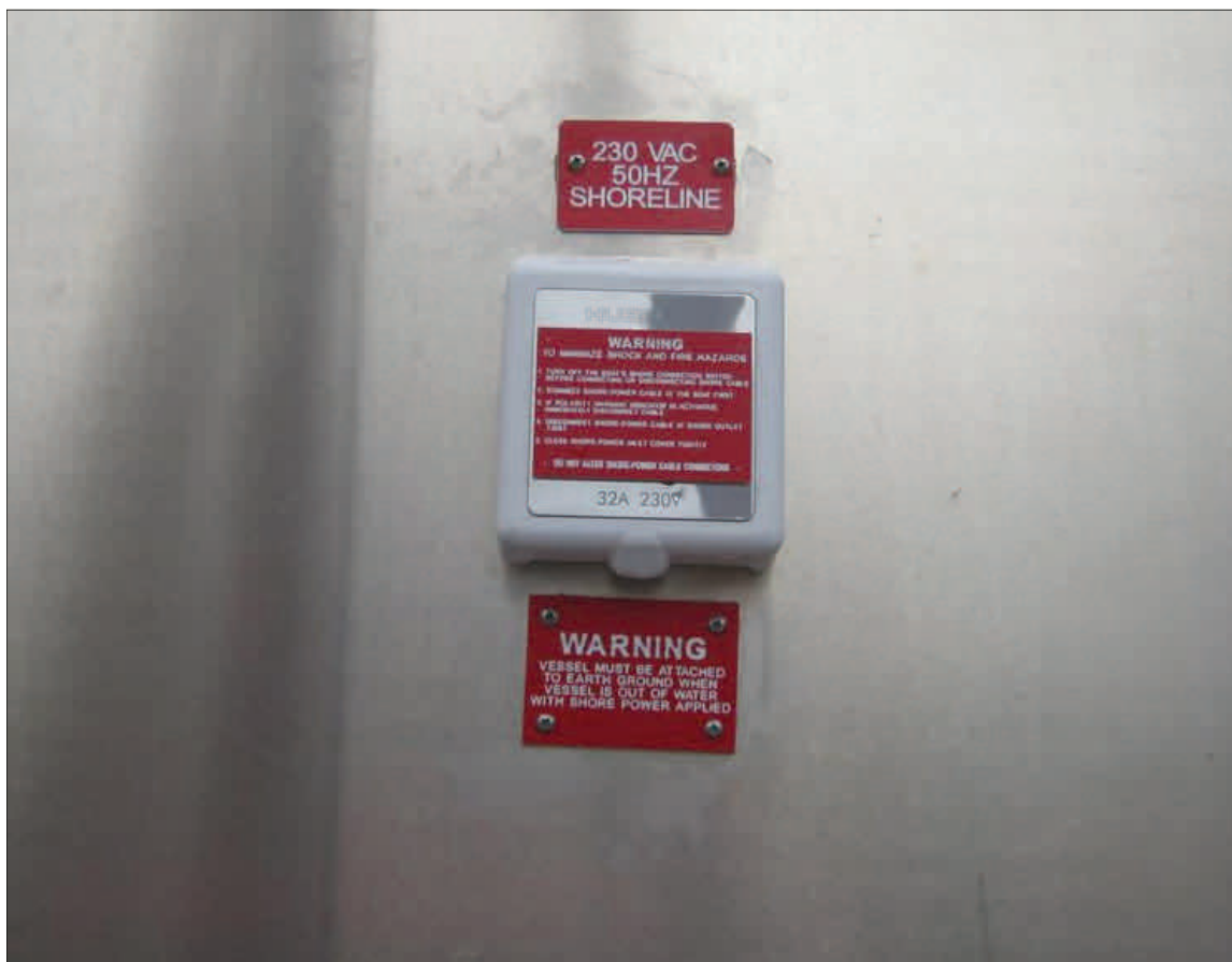
Figure 311-3a. Example Shore Power Connection
